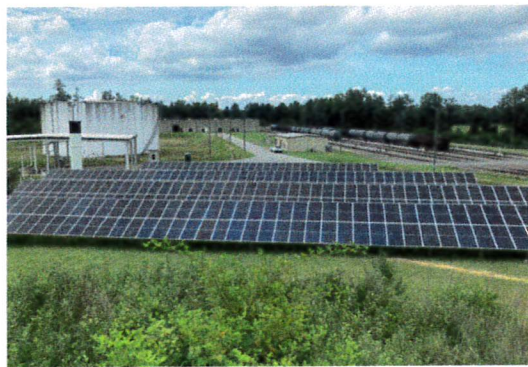
Eco Energy Augusta, 152 kW, 2021
