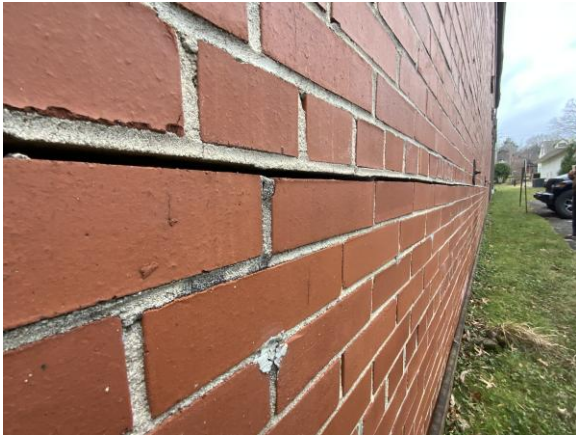
Photo 13: North wall horizontal crack.
