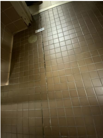
Photo 19: Crack in slab.
