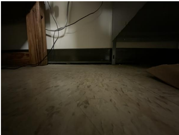
Photo 25: Gap between slab and cove base.
