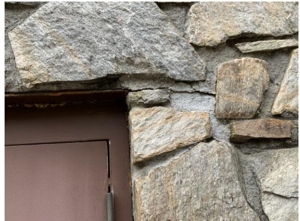
Photo 34: Cracked stone veneer.
