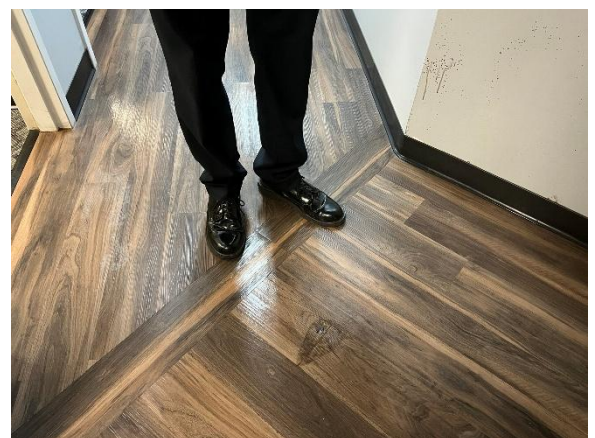
Photo 7: Water intrusion near detective office.
