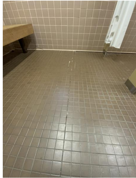
Photo 18: Crack in slab.
