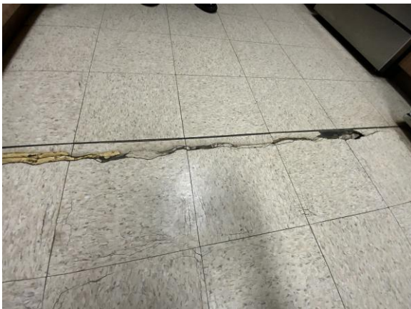
Photo 15: Differential settlement in slab.
