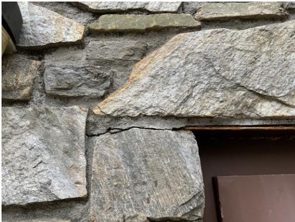
Photo 33: Cracked stone veneer.
