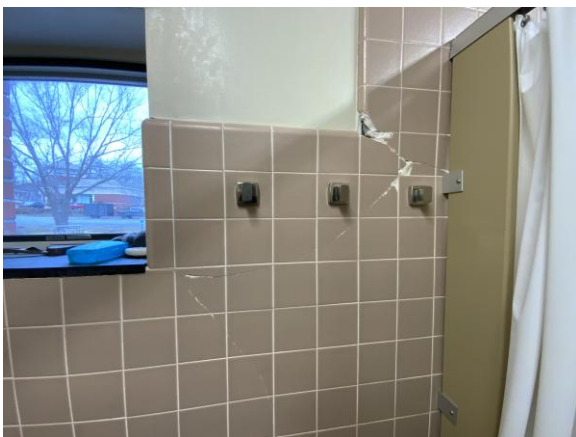
Photo 21: Cracks in wall tile.
