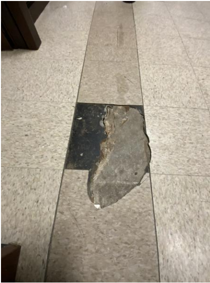
Photo 17: Crack in slab.
