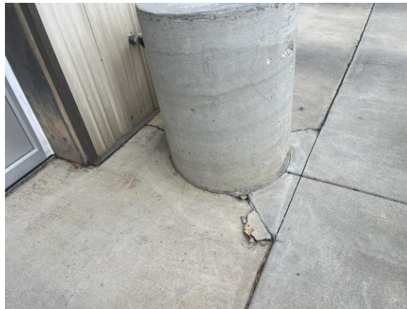
Photo 3: Settlement near apparatus bay.
