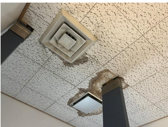
Photo 6: Water damage in police station bathroom.
