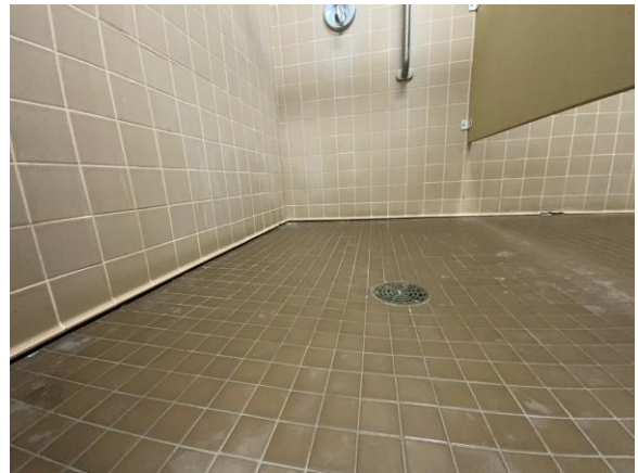
Photo 26: Gap between slab and cove base.
