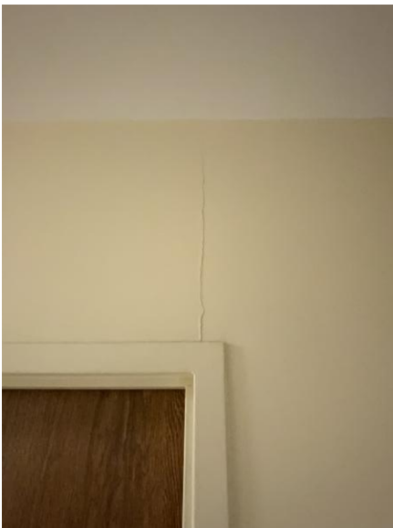
Photo 27: Crack in gypsum board.
