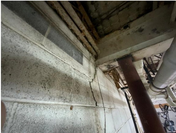
Photo 10: East wall separation from building.
