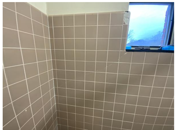
Photo 22: Cracks in wall tile.
