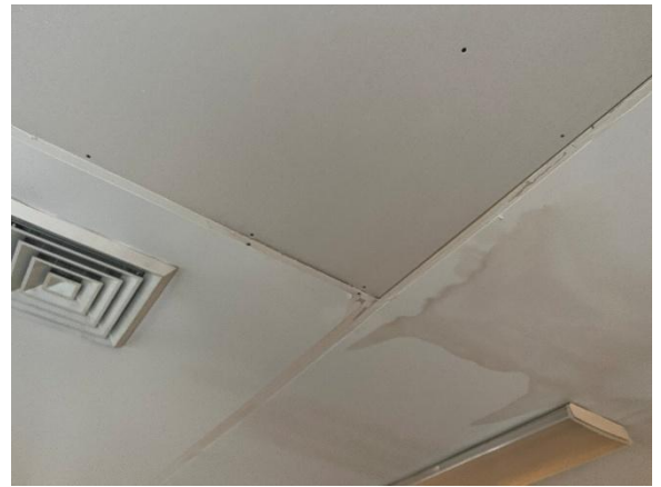
Photo 5: Water damage in fire station living room.
