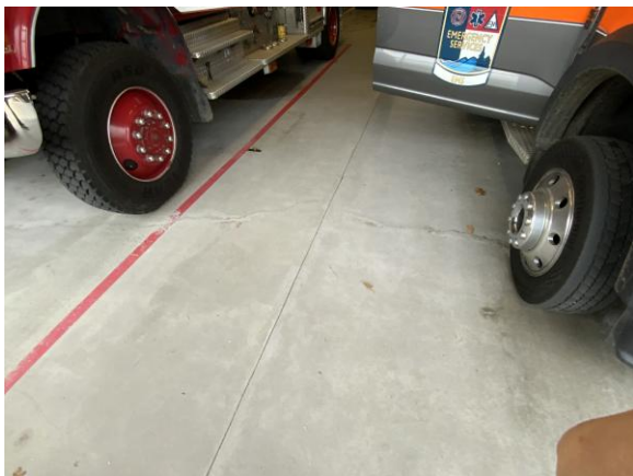
Photo 35: Apparatus bay slab crack.
