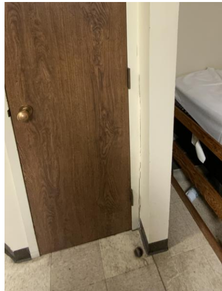
Photo 20: Cracks in gypsum board.
