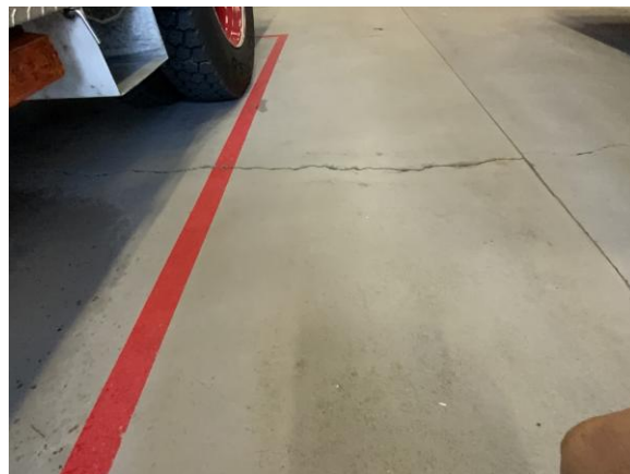
Photo 36: Apparatus bay slab crack.
