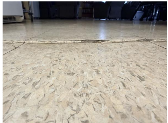
Photo 16: Differential settlement in slab.
