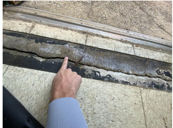
Photo 14: Differential settlement in slab.
