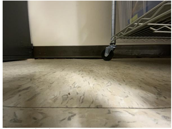
Photo 24: Gap between slab and cove base.
