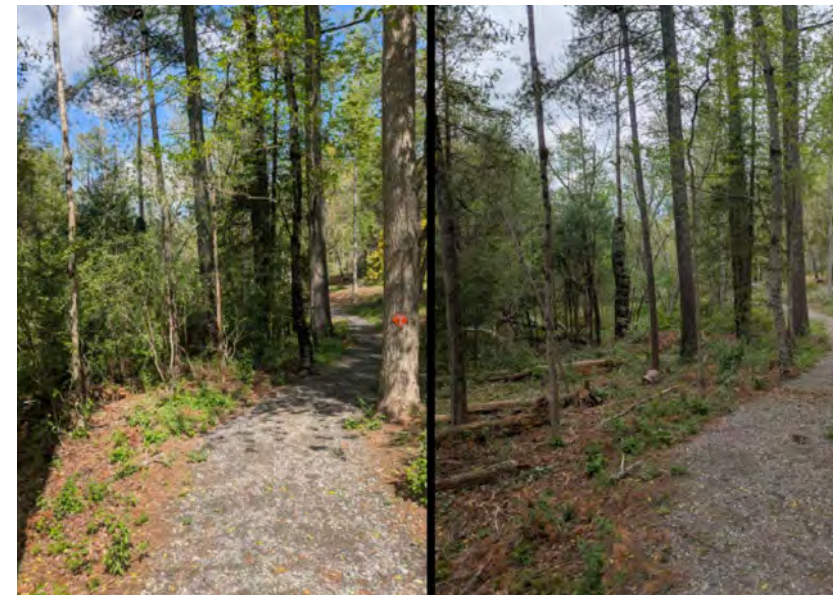
NNIS Removal for Stream Restoration Project_Before and after cut stem treatment – mostly autumn olive and Chinese privet.
