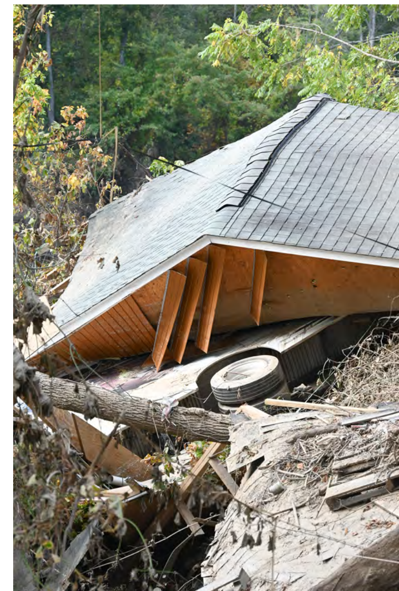
Home damaged beyond repair.
