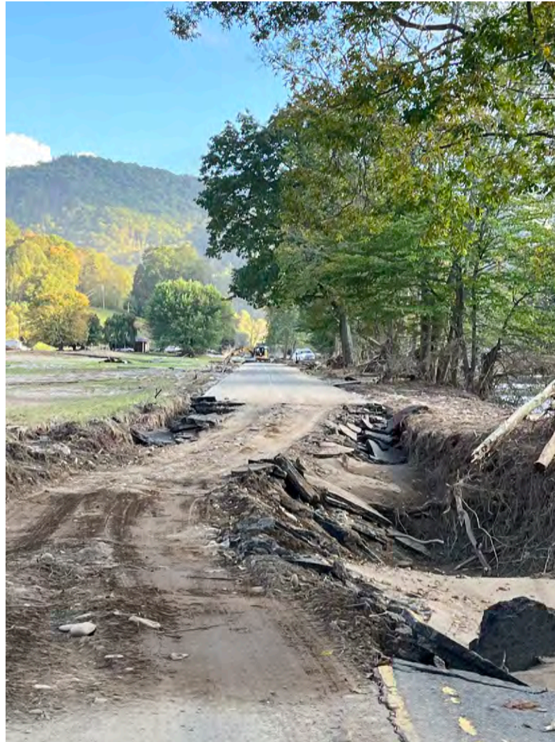
Damaged Roads: limit residents on transit options.
