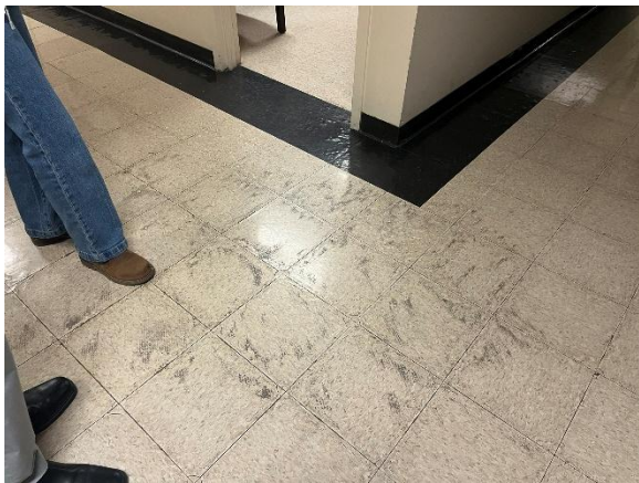
Photo 16: Damaged VCT in corridor.
