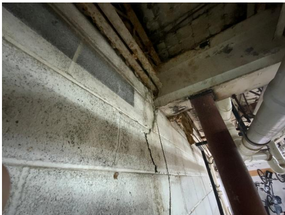
Photo 77: East wall separation from building.
