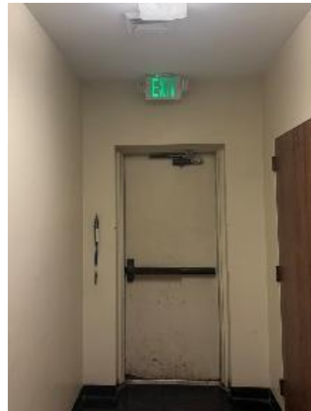
Photo 50: Egress light fixture.
