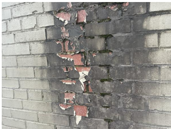
Photo 7: Peeling paint below downspout opening.
