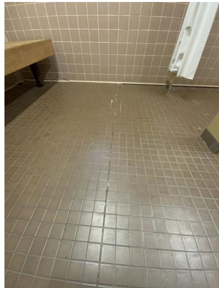
Photo 85: Crack in slab.
