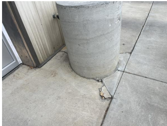
Photo 23: Settlement near apparatus bay.
