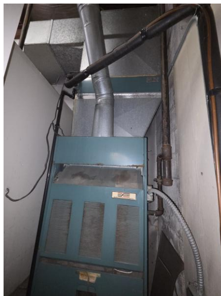
Photo 38: Gas furnace serving truck repair room.
