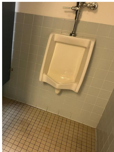
Photo 62: Manual flush valve urinal.
