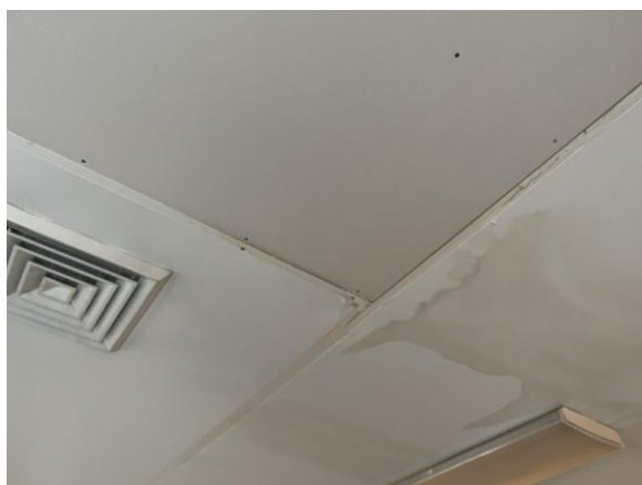
Photo 10: Water damage in fire station living room.
