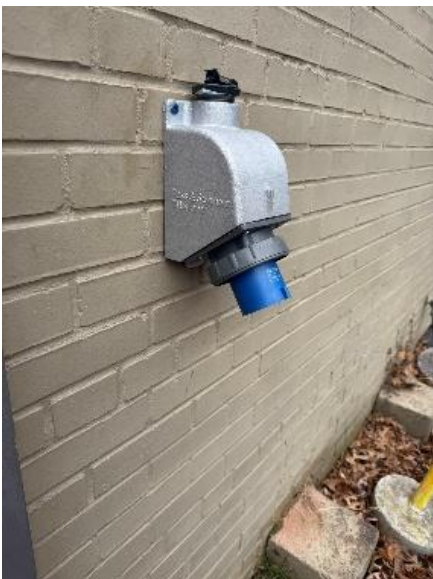
Photo 45: Portable generator connection.
