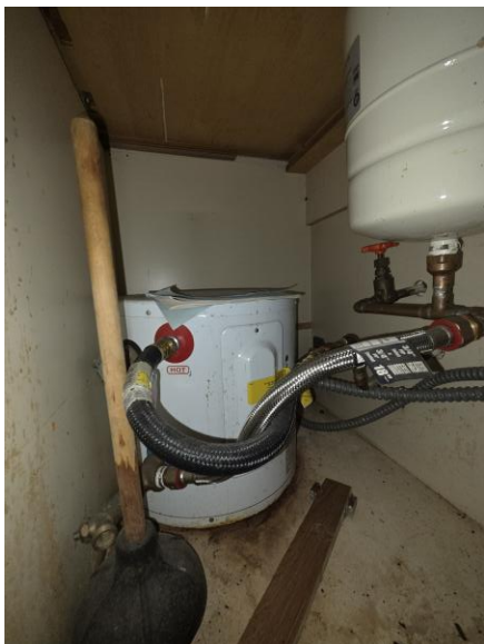
Photo 71: Mini-tank water heater.
