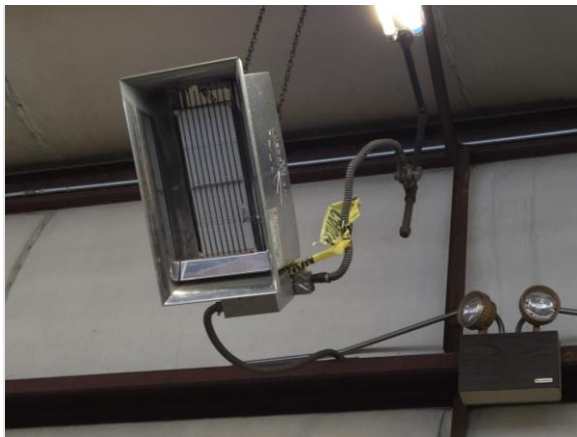
Photo 35: Electric unit heater.
