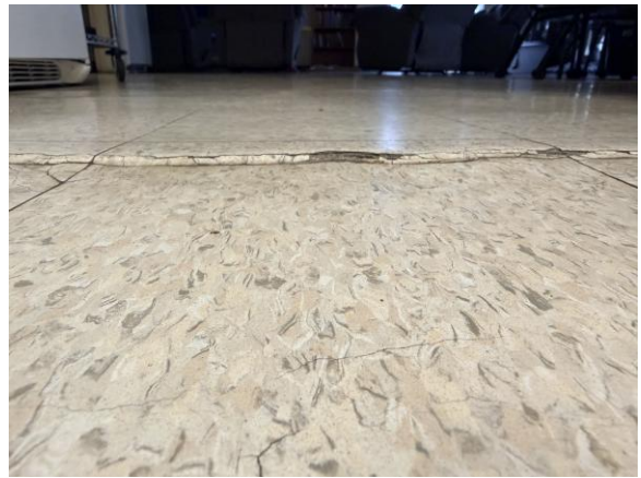
Photo 83: Differential settlement in slab.
