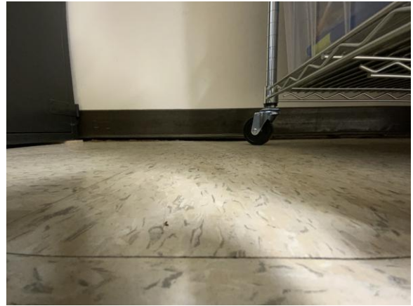
Photo 91: Gap between slab and cove base.
