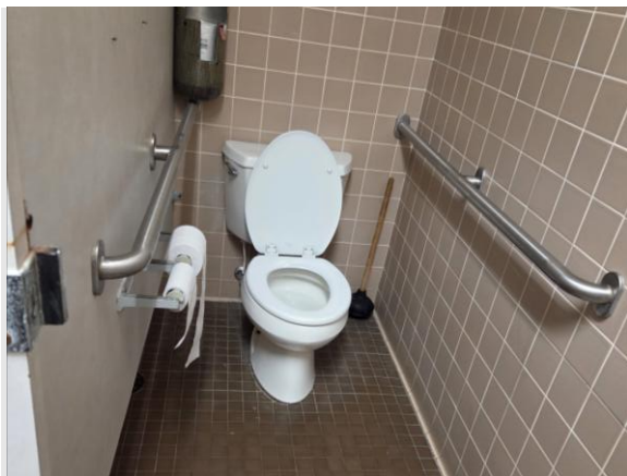
Photo 67: Tank type water closet.
