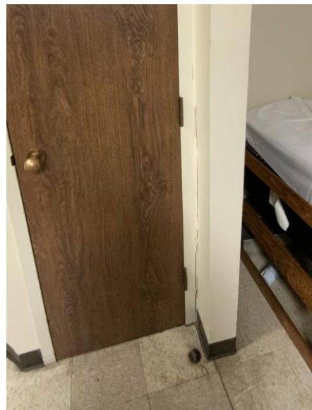
Photo 87: Cracks in gypsum board.
