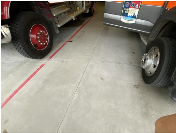
Photo 102: Apparatus bay slab crack.
