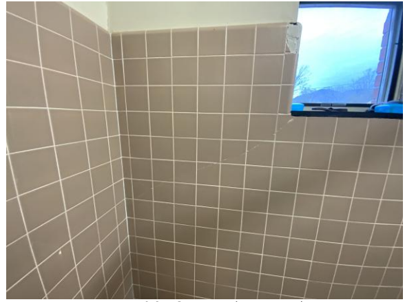
Photo 89: Cracks in wall tile.
