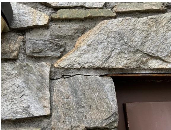
Photo 100: Cracked stone veneer.
