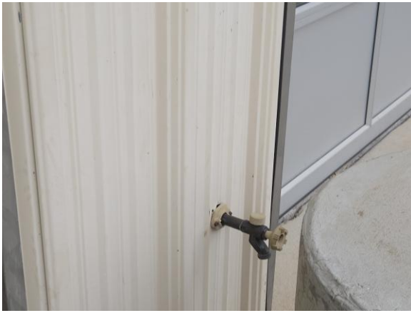
Photo 73: Fire station exterior hose bibb.
