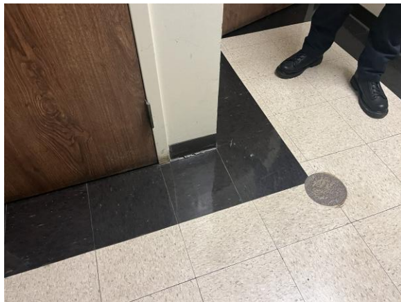
Photo 17: VCT with water intrusion.
