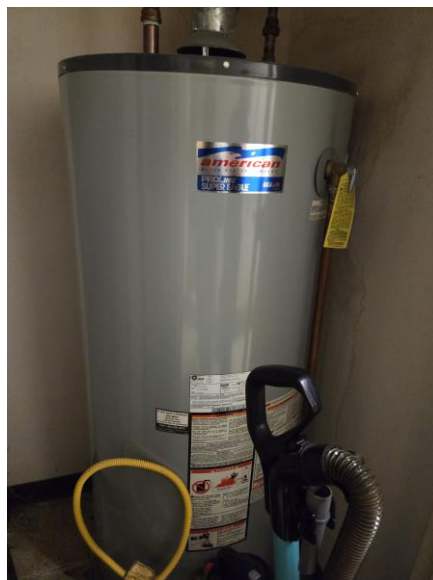
Photo 70: Storage room water heater.
