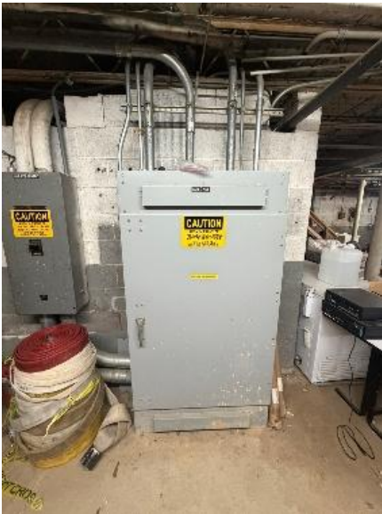
Photo 41: Main disconnect and MDP.
