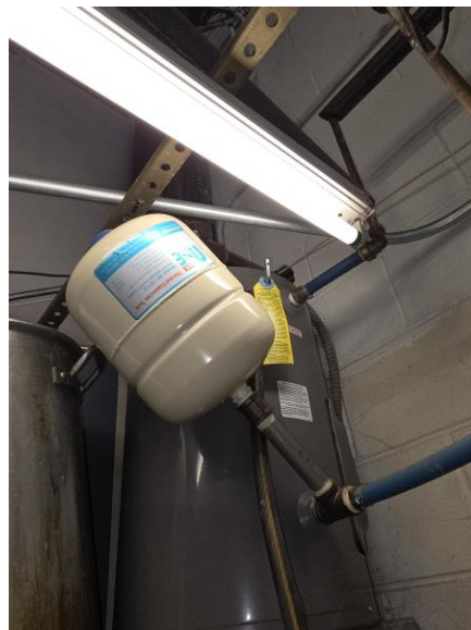
Photo 72: Fire station area water heater.
