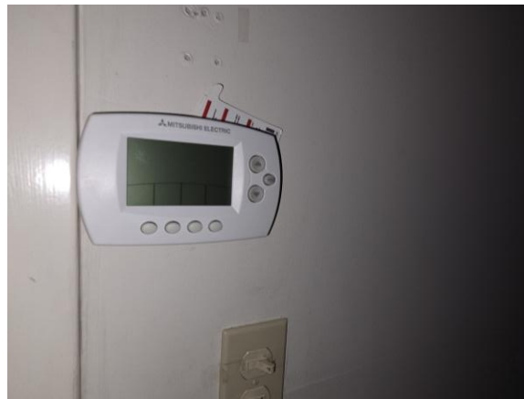
Photo 28: Nonfunctional IT room thermostat.
