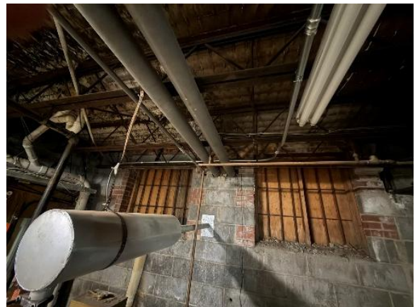
Photo 40: Electrical service routing in basement.
