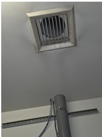
Photo 29: IT room exhaust fan.
