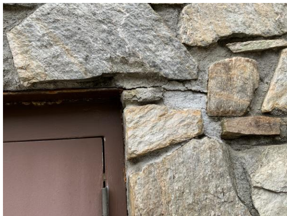
Photo 101: Cracked stone veneer.
