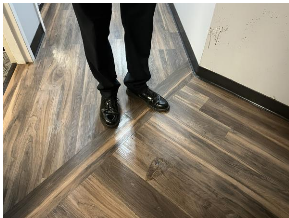
Photo 20: Water intrusion near detective office.
