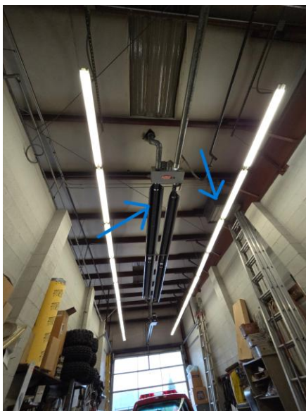
Photo 37: Maintenance room infrared heater and exhaust fan.
