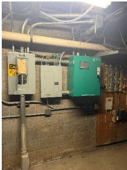
Photo 44: Automatic transfer switch.
