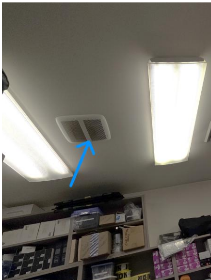
Photo 31: Equipment room exhaust fan.
