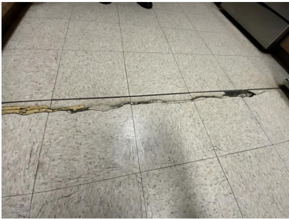
Photo 82: Differential settlement in slab.
