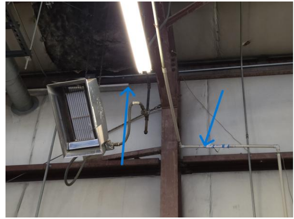
Photo 74: Disconnected water piping.
