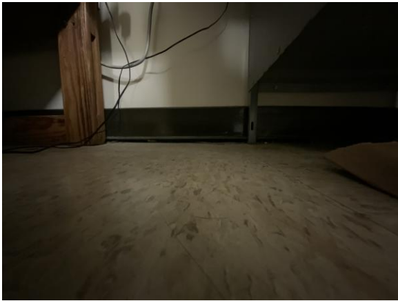
Photo 92: Gap between slab and cove base.
