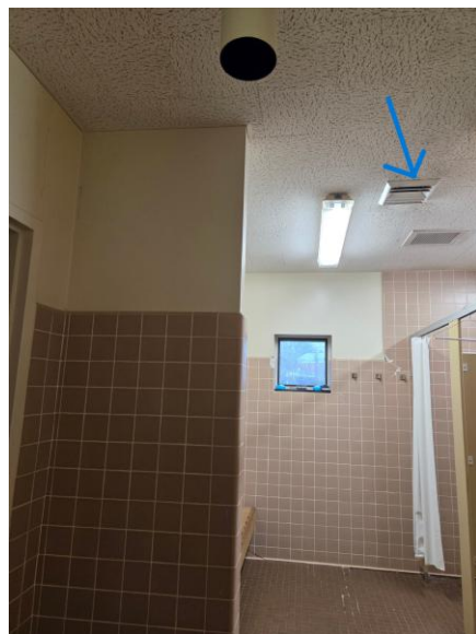
Photo 34: Men's restroom shower exhaust fan.
