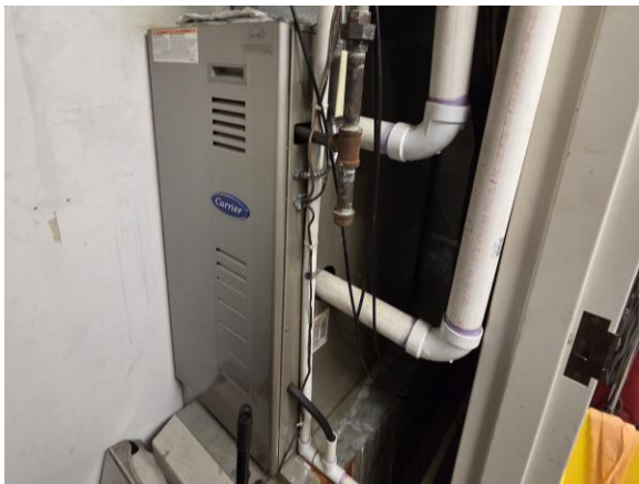
Photo 27: Typical furnace serving police department.
