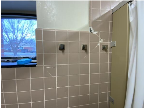
Photo 88: Cracks in wall tile.
