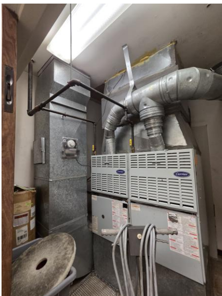
Photo 33: Gas furnace serving fire station.
