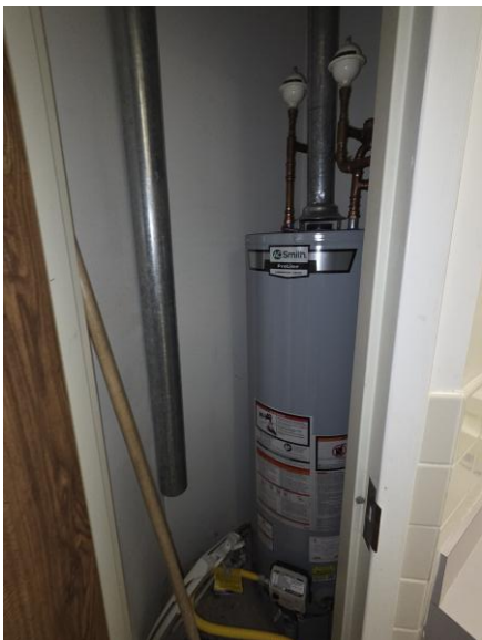
Photo 65: Water heater inside restroom closet.
