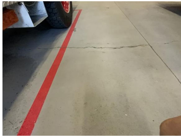
Photo 103: Apparatus bay slab crack.
