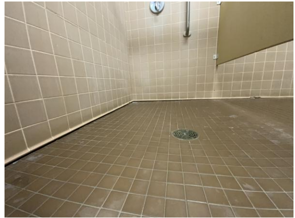
Photo 93: Gap between slab and cove base.
