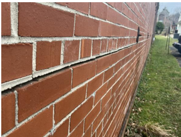
Photo 3: Mortar separation in north wall.
