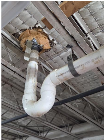
Photo 54: Crumbling ceiling at P-trap.
