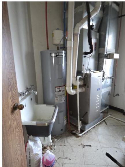
Photo 66: Water heater in mechanical room.
