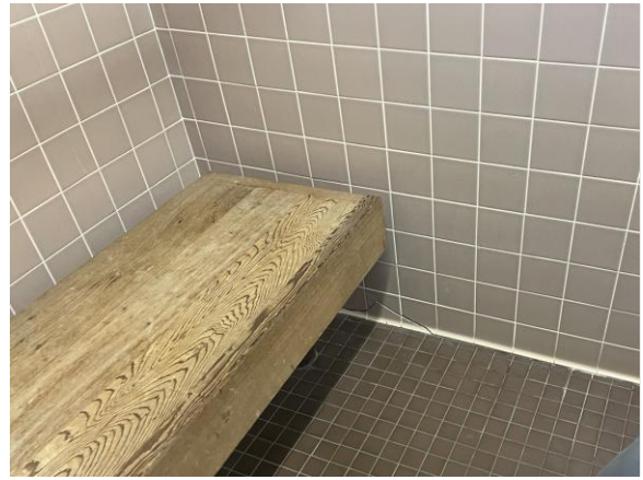
Photo 13: Cracked tile in shower.
