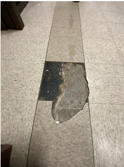
Photo 84: Crack in slab.
