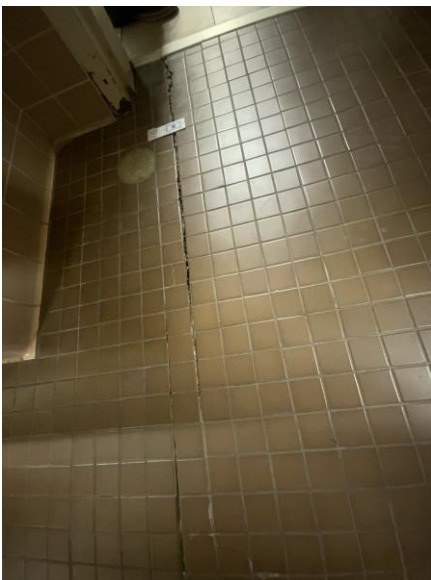
Photo 86: Crack in slab.
