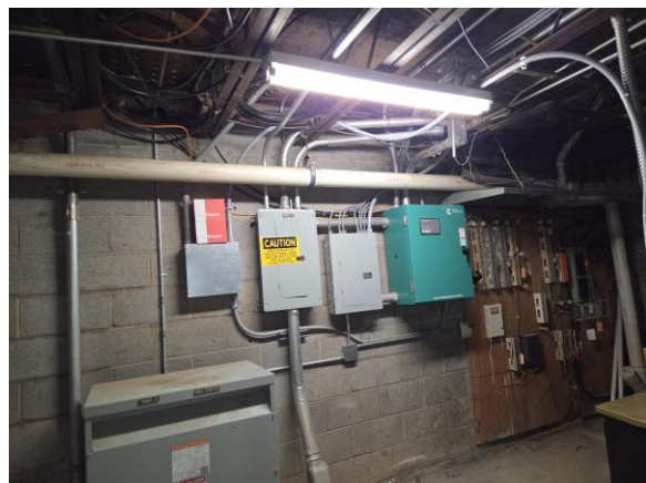
Photo 60: Sanitary piping above electrical panels.
