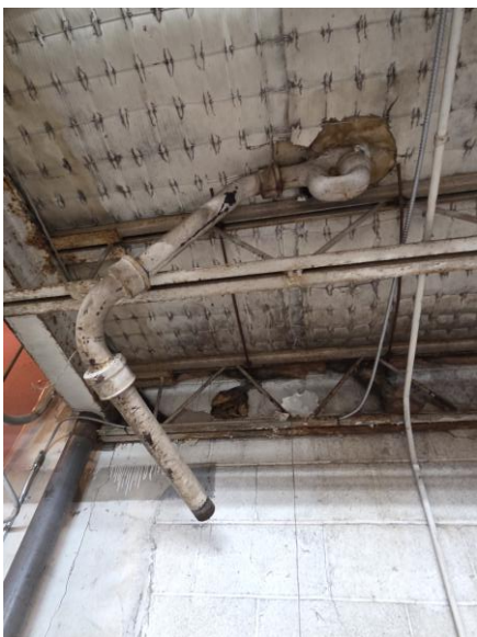
Photo 55: Open-ended sanitary waste piping.
