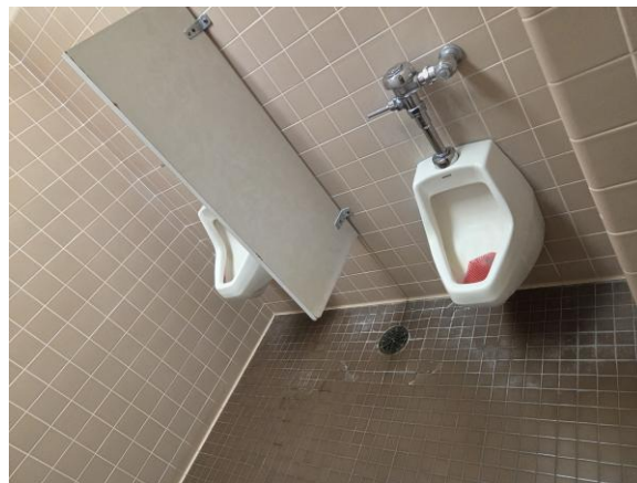
Photo 68: Manual flush valve urinal.
