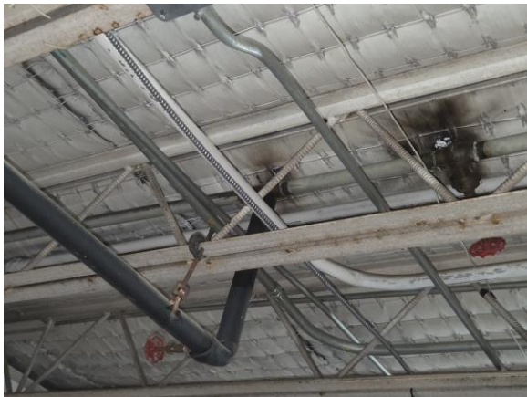
Photo 57: Uninsulated water piping.
