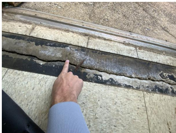
Photo 81: Differential settlement in slab.
