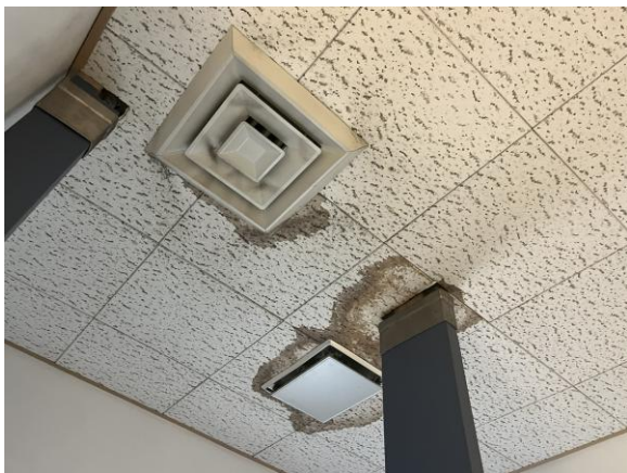
Photo 19: Water damage in police station bathroom.
