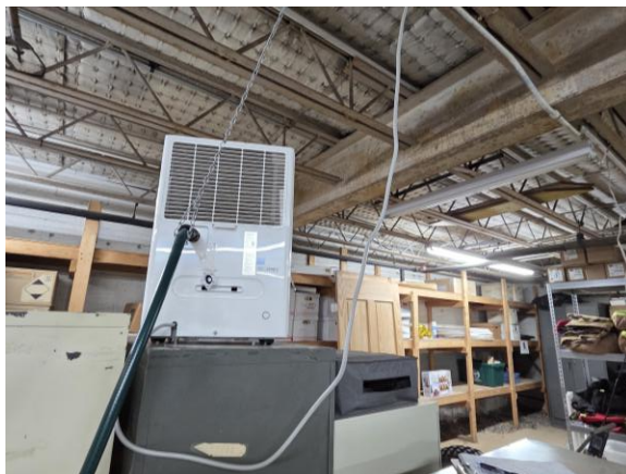
Photo 24: Dehumidifier serving police department basement.
