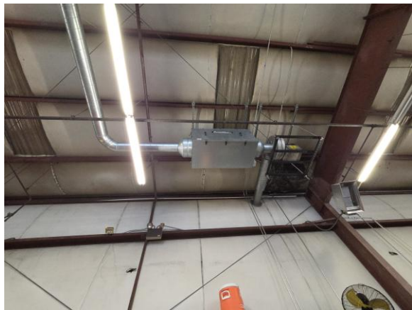
Photo 36: Vehicle exhaust extraction unit.
