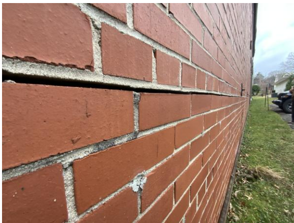
Photo 80: North wall horizontal crack.
