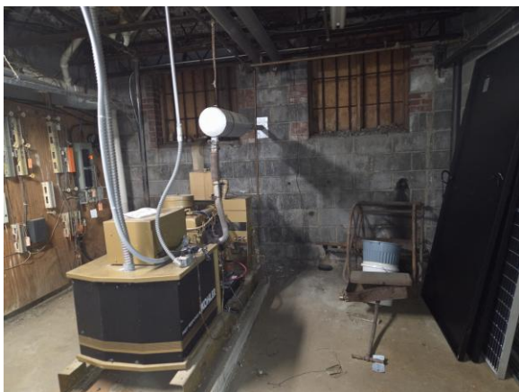
Photo 59: Generator and uninsulated piping.
